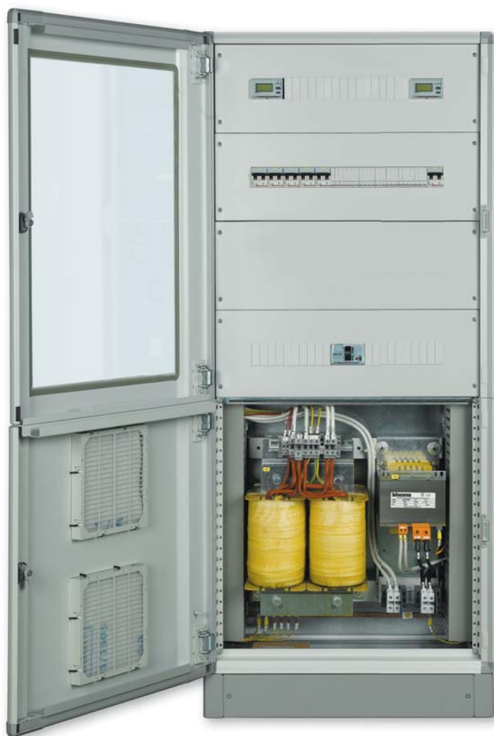
Distribution board with insulation and safety transformer
